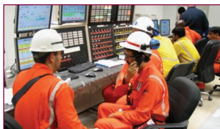
QG2 Inlet Receiving Main Control Room (MCR)
