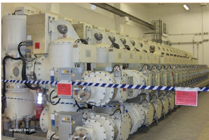
66KV GIS at SS-2901
