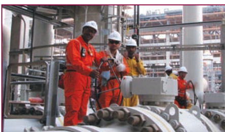
Personnel open valves to introduce gas into Inlet Receiving
